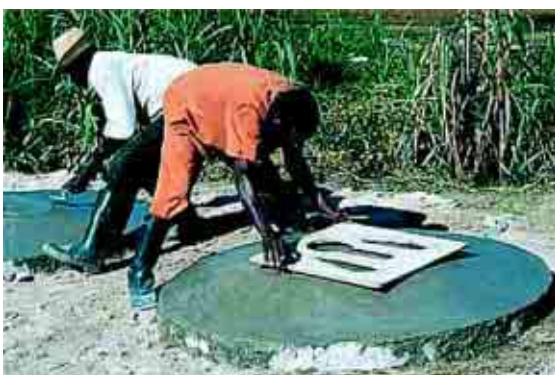
Figure 6. Concrete slabs constructions for latrines. In: National Programs of Sanitation in Mozambique: Pioneer in the Suburban Sanitation , 2002, p. 01. {www.wsp.org}.
