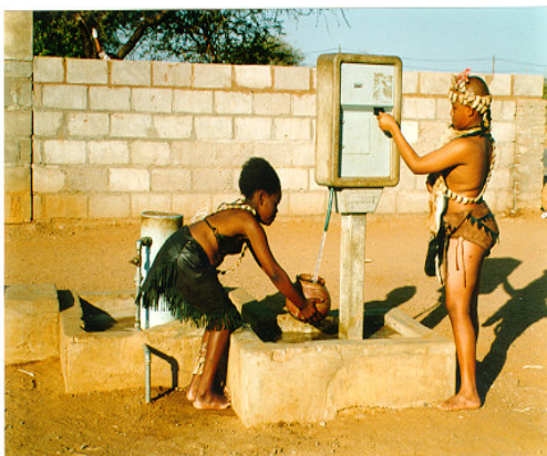
An installed prepaid meter system in operation.
