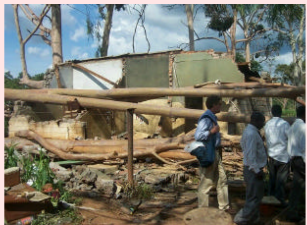
This house in Kadoma was completely destroyed by a hailstorm
